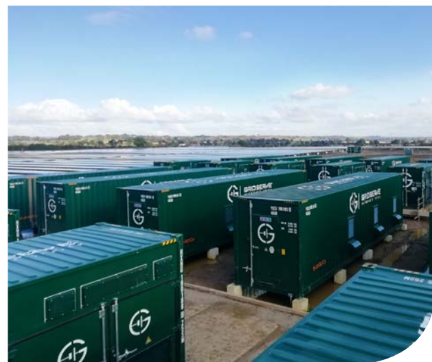
27.5MW/30.14MWh PV+ESS Yorkshire, England 🇬🇧
